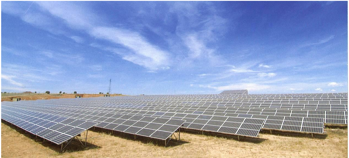
Figure 1: Typical solar panel farm
