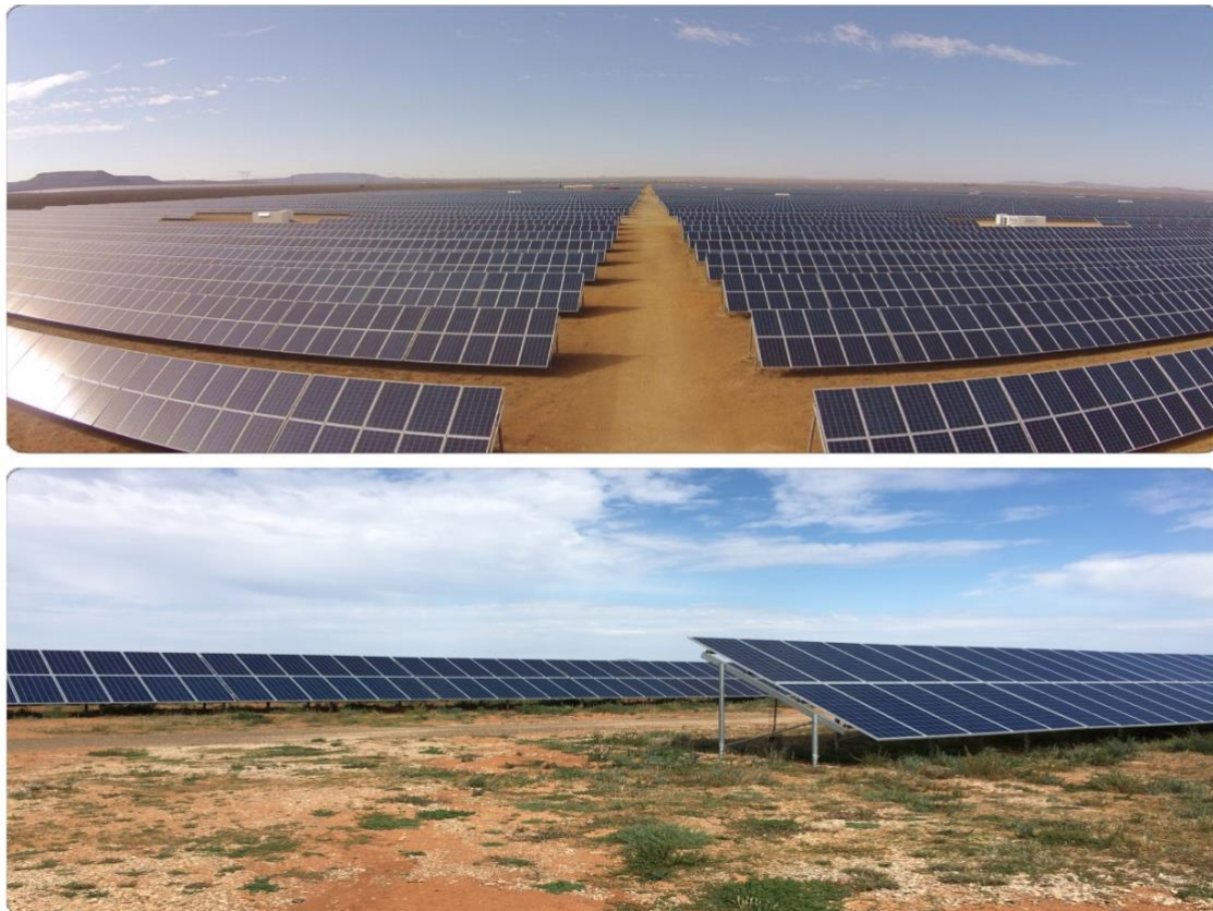
Figure 2-1: Photo showing an elevated view of PV panels & from ground level
