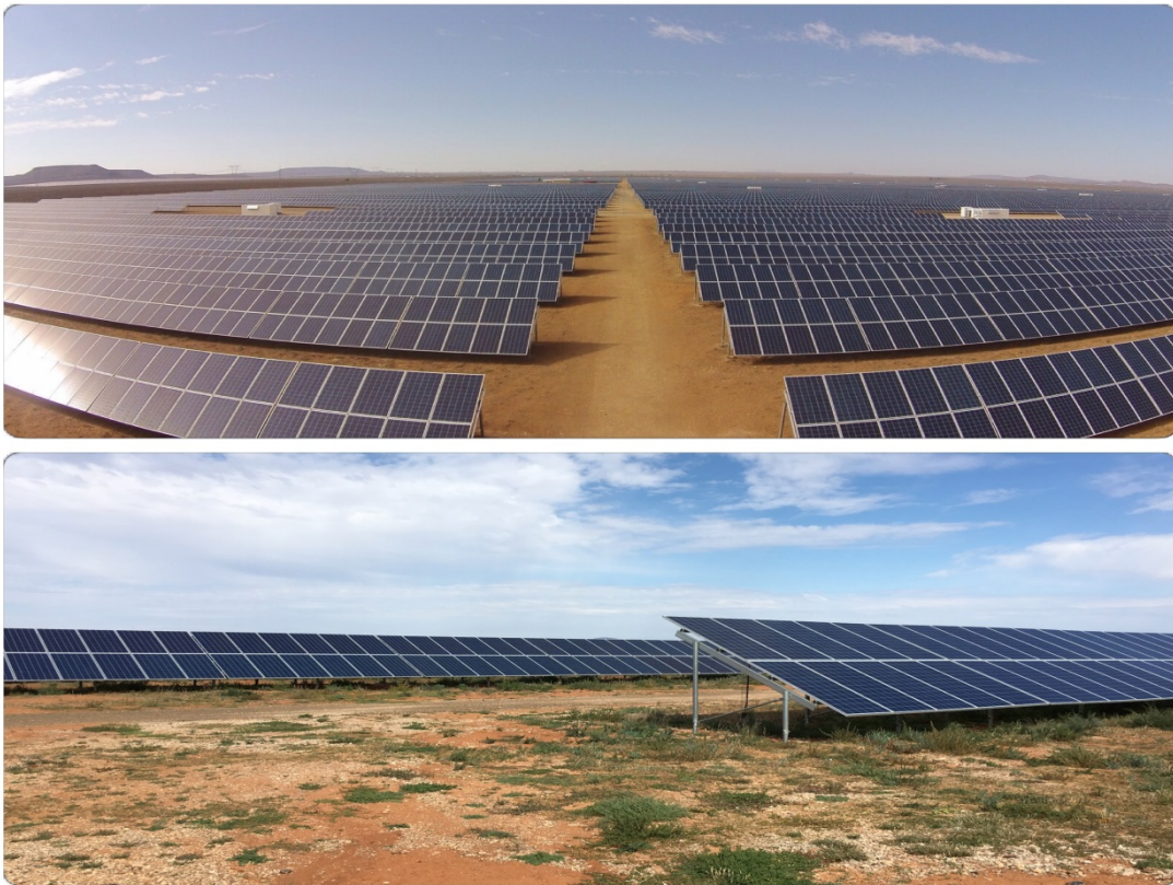
Figure 2: Photo showing an elevated view of PV panels & from ground level
